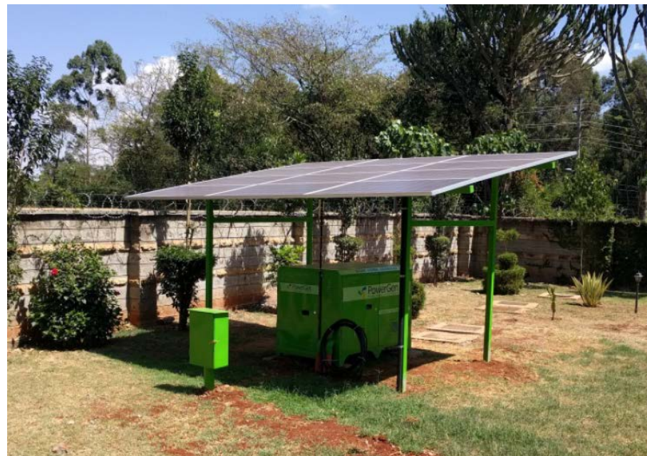
PV mini-grid station by Powergen: Kenya
