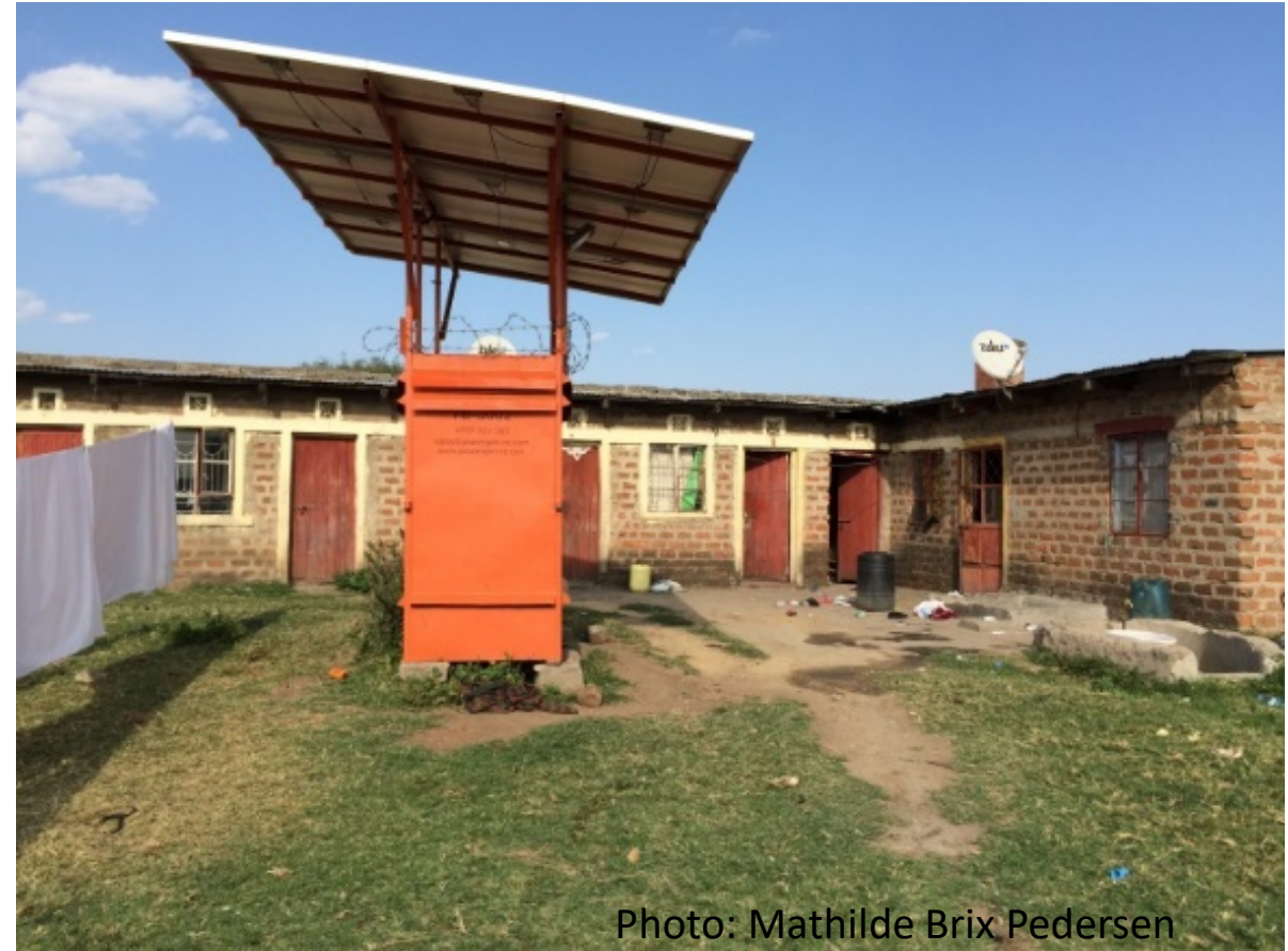
1.4 kW mini-grid, PowerGen
